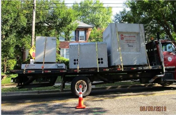
Tap hole, Transformer Enclosure, & Manhole
